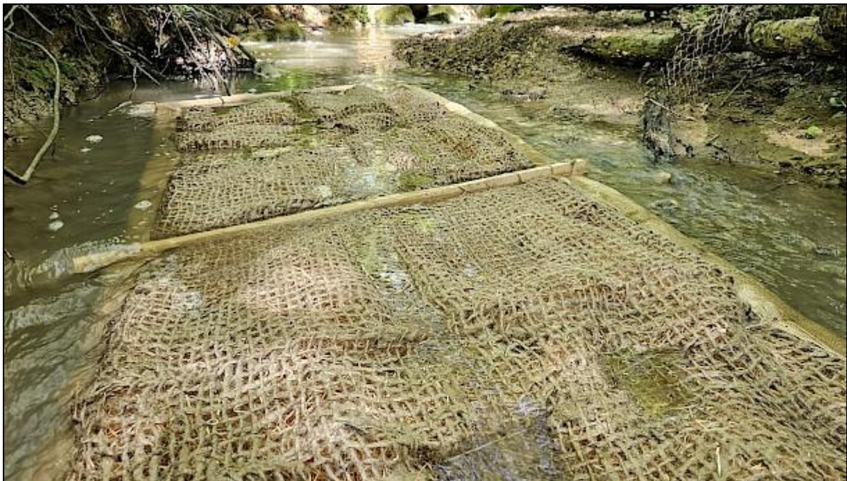
Figure 5-7 – Typical Sedimat Installation
